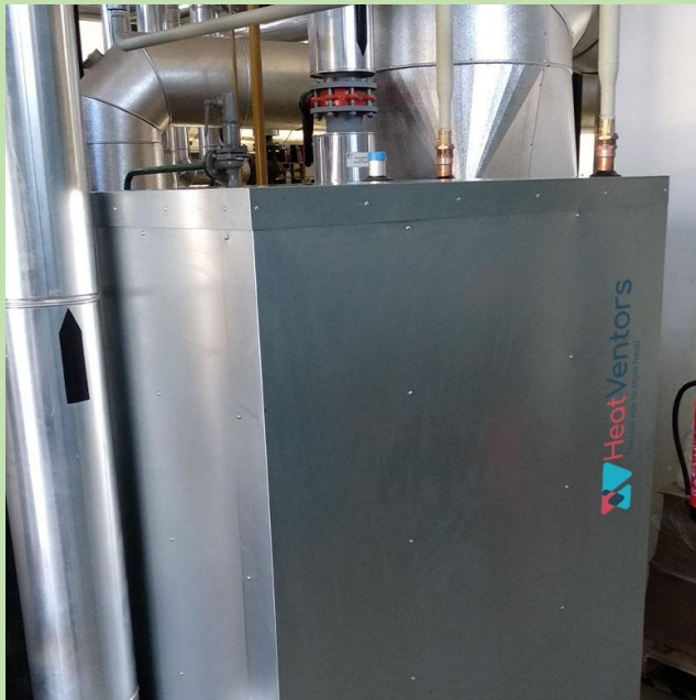
Heat exchanger + insulated box
